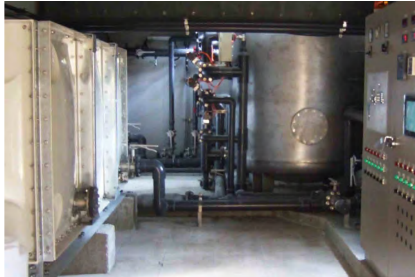
The raw water treatment systems
